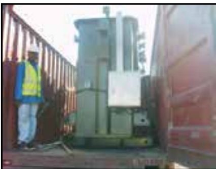
20kV Glad Mine installation
